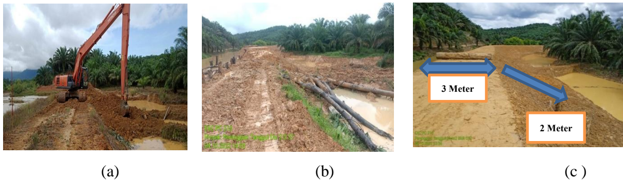
Figure 5: Heightening of banks along the rivers (a) works by excavators, (b) embankment in progress and (c) completed embankment with 3 meter width on the top surface
